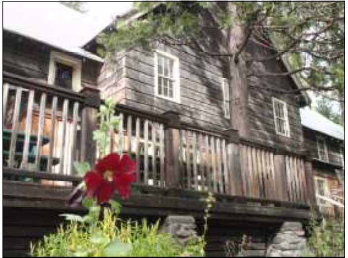
The Main Lodge at Breitenbush remains standing while a new foundation is being constructed.
